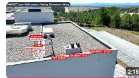
OAIBOX Open RAN - Testing Network Slicing 1k views • 1 year ago
